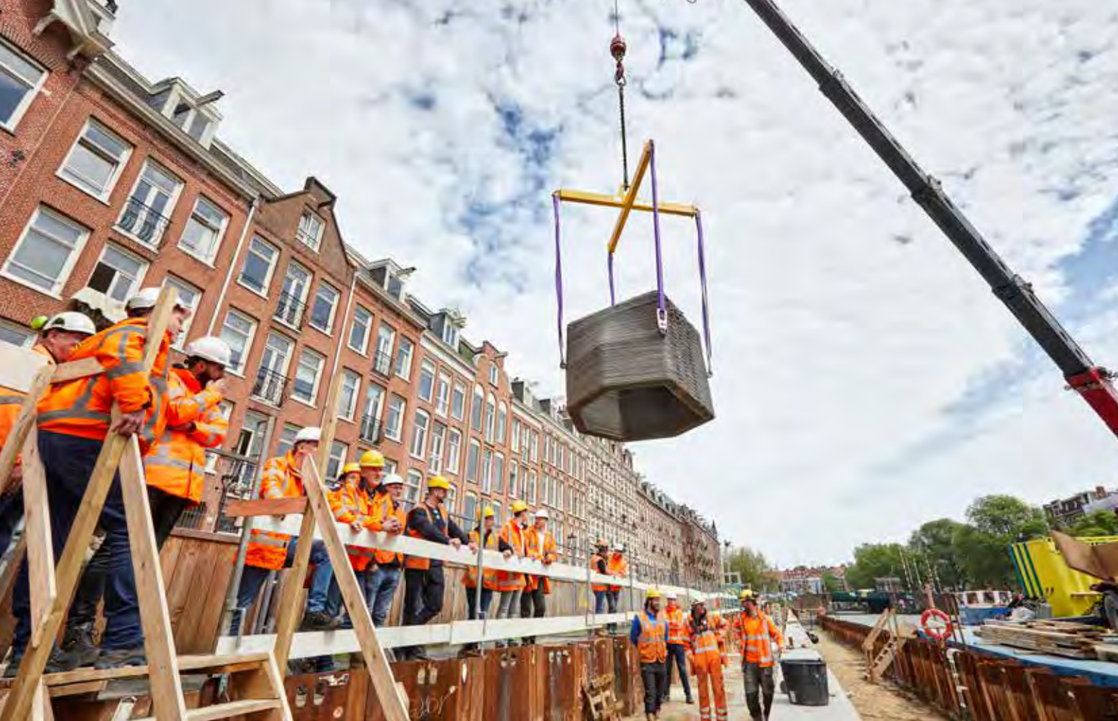
Placement of 3D-printed canal wall pit sheets at the Jacob Catskade-project in Amsterdam, in collaboration with Neolithic.
